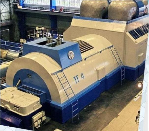
Turbogenerator at CHPP
