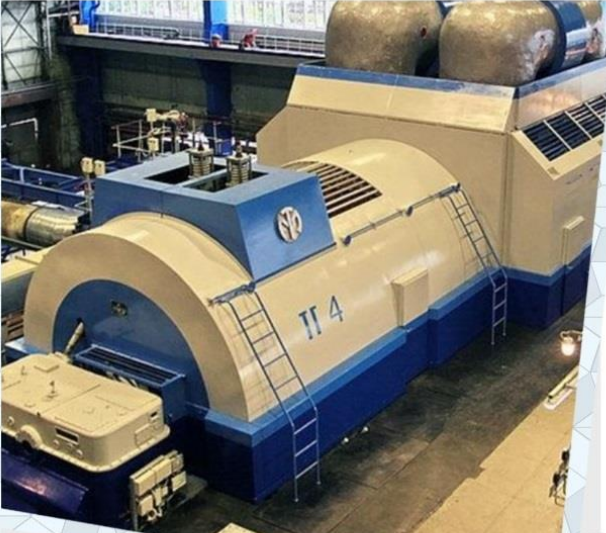
Turbogenerator at CHPP
