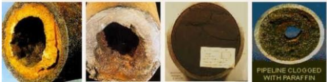
Figure 20.2 – Paraffin plugs in the oil pipeline
